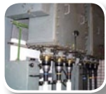
Power sensitive equipment
