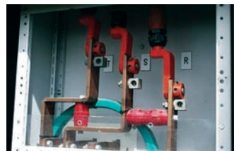
Insulated rotary clamps provided a compact connection to slotted busbar
