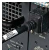
Electrical Infrastructure Labeling
