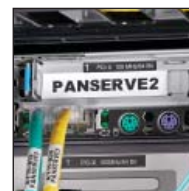
Network Infrastructure Labeling
