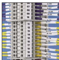
Terminal Block Labeling
