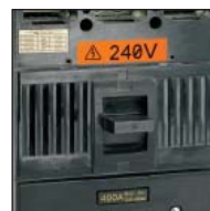
Electrical Hazard Labels
