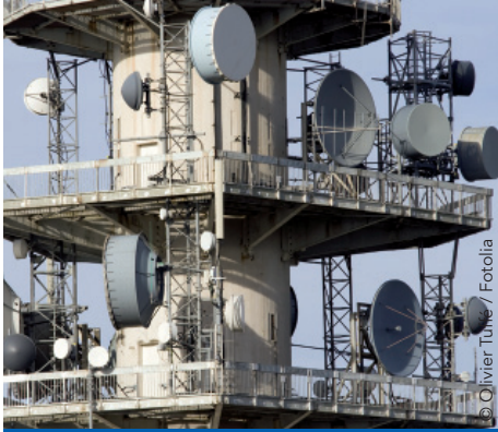
Telecom - Data infrastructure
