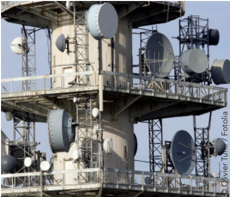
Telecom - Data infrastructure
