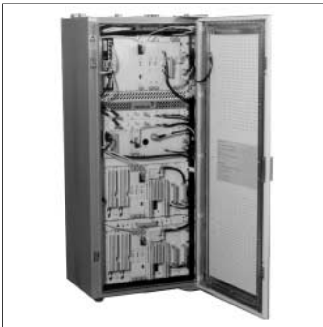
Base station of cellular network
