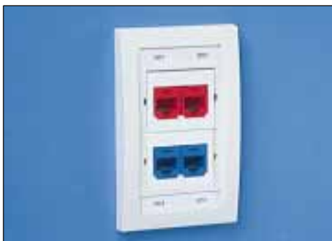
Network Systems Labeling
