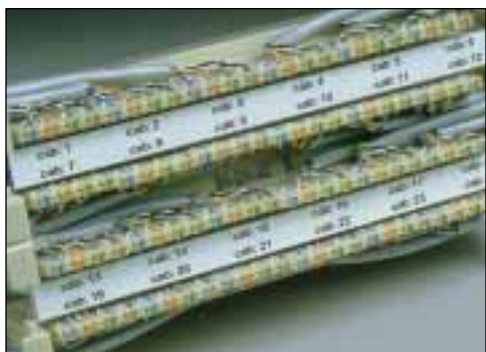
Network Systems Labeling
