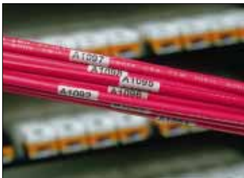
Wire and Cable Identification
