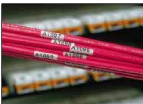
Wire and Cable Identification
