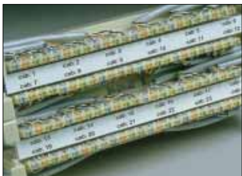
Network Systems Labeling
