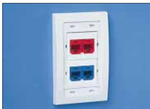
Network Systems Labeling
