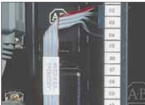
Terminal Block Labeling
