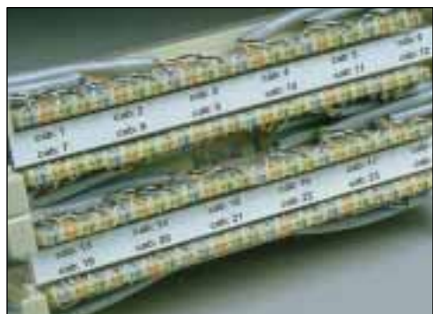
Network Systems Labeling
